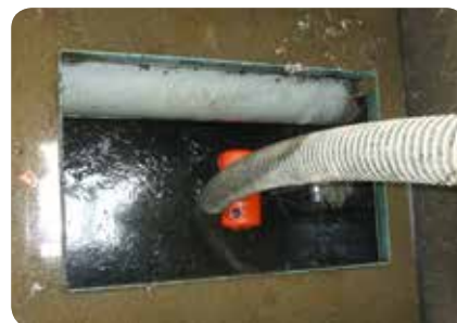
View of the separator chamber
