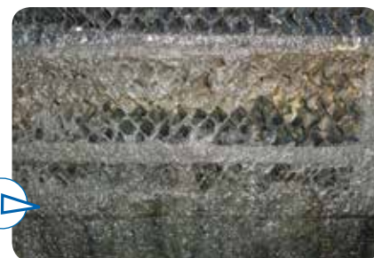
Detail of a coalescing filter heavily loaded in sludge and requiring intervention.
