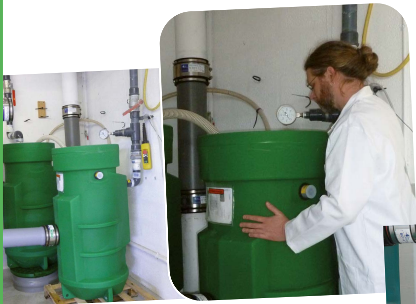
Testing basis: verification of a pumping station's performance
