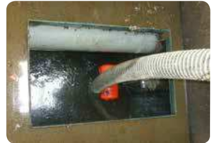
View of the separator chamber
