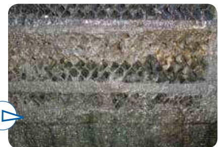
Detail of a coalescing filter heavily loaded in sludge and requiring intervention.
