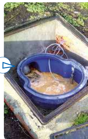
Example of a grease separator which requires emptying
